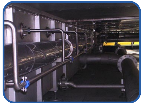
CIP Pipe work
